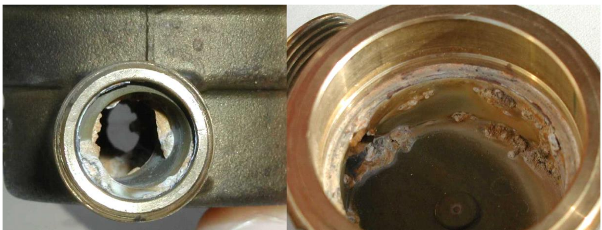
Figure 4. Limescale built-up in the inside of a single jet water meter housing
