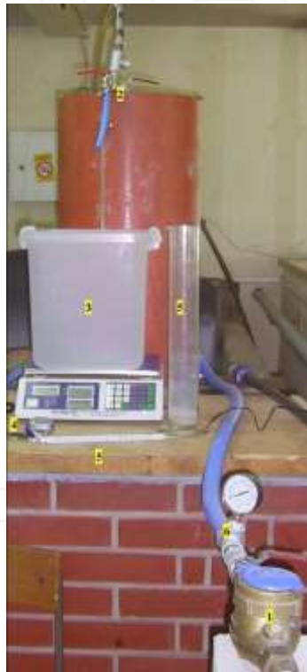
Figure 3. Part of the water supply pipeline downstream from the water meter (1) in the Hydraulic Laboratory of the Faculty of Civil Engineering in Subotica. 2 - stop valve, 3 - vessel with scale for measuring water quantity flown through the water meter, 4 - stop-watch, 5 - measuring cylinder and thermometer, 6 - manometer.
